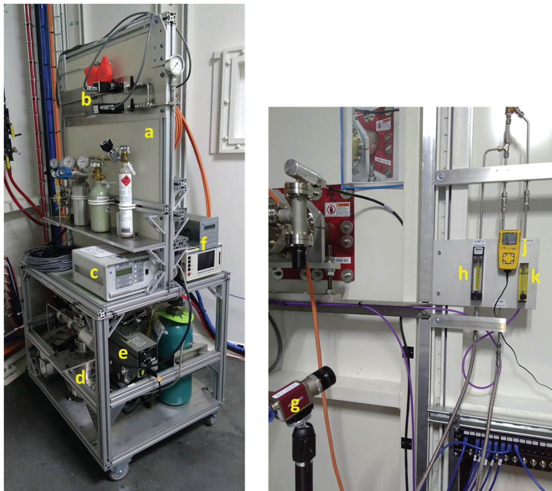
Figure 4: Integrated gas inlet and gas analysis system (left) and exhaust system (right) at QAS: (a) gas cart (flammable side); (b) mass flow controllers (MFCs); (c) MFC electronics; (d) residual gas analysis (RGA) turbomolecular pump; (e) RGA head and electronics; (f) turbo pump controller and pressure readout; (g) camera; (h) gas outlet flowmeter; (i) multiple gas environment monitoring device; (k) nitrogen flowmeter.
