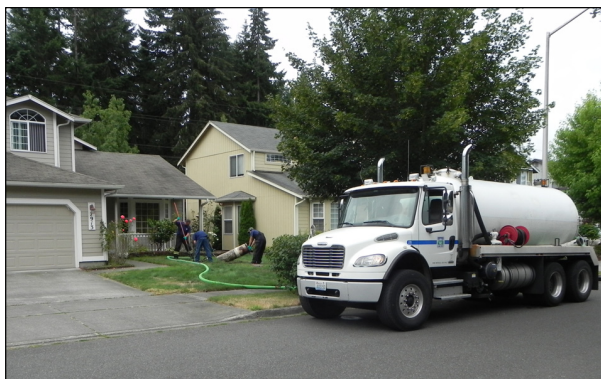
In 2008, Lacey adjusted its STEP maintenance to reduce unnecessary costs, including changing tank pump-outs to an eight-year schedule.
