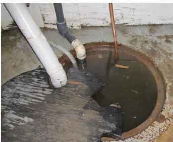
**Alstadt and Morris 11/12/12, Poughkeepsie flooded pump well
