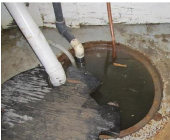
*Alstadt and Morris 11/12/12, Poughkeepsie flooded pump well
