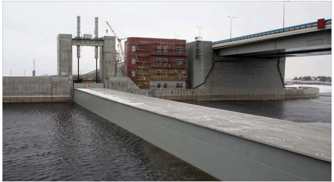
Cut off: The barrier gate in position at navigation S1. It is lifted by four hydraulic cylinders
